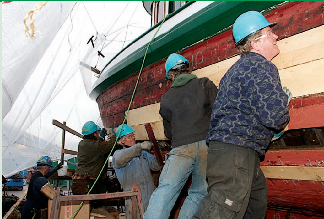
Matthew Carruthers , right, and Sean Bull , lean into the plank to bend it into place while Dave Lyng uses a large clamp to secure it.
