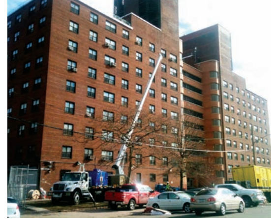
A Foss crew used a boom truck to supply water to the main building at the Ocean Bay Apartments in Queens, N.Y., which in turn supplied water to the entire complex of 26 buildings operated by the New York City Housing Authority.
